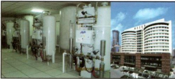
Shanghai East Hospital (Tongi University) China A 1500 Bedded Hospital having equivalent 375 D Type oxygen Cylinder capacity - AS-L Triplex system running since 2008
