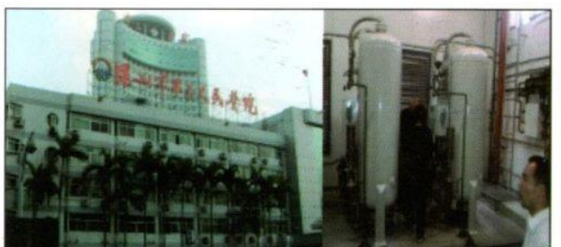
Shenzhen futian District people's hospital, china With 1250 Bedded, A 24 floors Hospital having equivalent 375 D Type oxygen Cylinder capacity - AS-L Triplex system running since 2003
