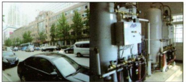
Jinzhou the first people's hospital, CHINA A 800 Bedded Hospital having equivalent 350 D Type oxygen Cylinder capacity - AS-N Duplex system running since 2003
