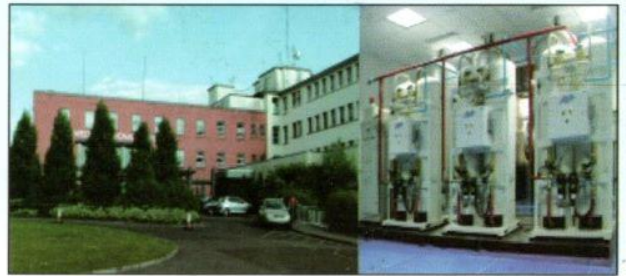
Limerick Hospital, Limerick, Ireland A 400 Bedded Hospital having equivalent 150 D Type oxygen Cylinder capacity - AS-J Triplex system running since 1997
